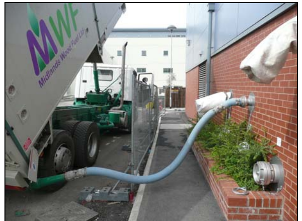
Delivering the commissioning load to a 500 kW boiler at a Manchester Hospital
