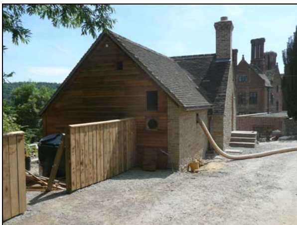
150 kW KOB chip boiler, installed at a country property in South Shropshire, by Intelligent Energy Ltd
