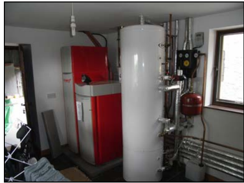
We have been pleased to support the customers of Intelligent Energy Ltd , a leading installer of 'Windhager' wood pellet boilers in the area.
