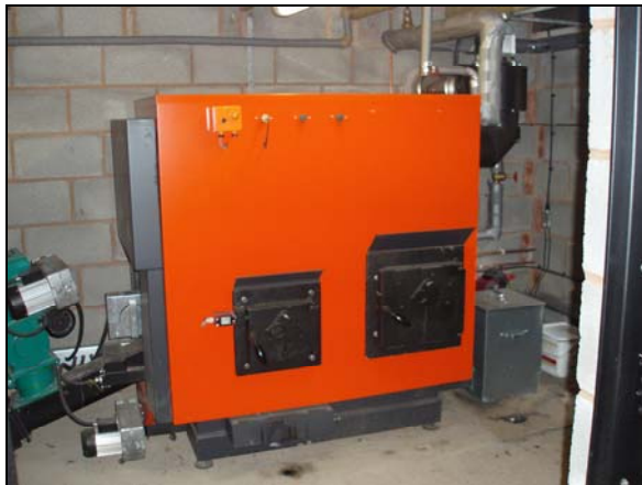
70 kW Heizomat chip boiler, installed by Mercia Energy Ltd at a site near Coventry.
