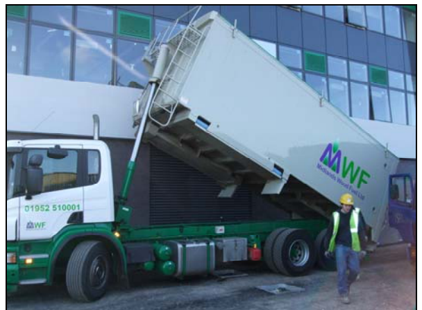
Delivery of the commissioning load of blown wood chips to the Froling 320 kW boiler installed by Econergy Ltd at Culcheth School, Warrington.
